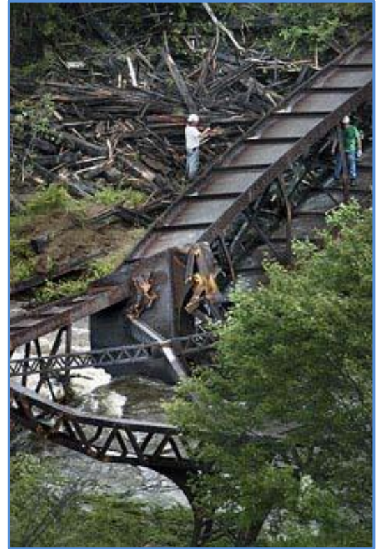
Engineers assess damage to the historic Kinzua Viaduct a day after a 1,400-foot section of the railroad bridge was ripped from its footings and dumped to the ground by an F1 Class tornado packing 100 mph winds.
